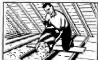
In attic with joists not of standard spacing, shows how to use Gold Bond Pouring Wool.
